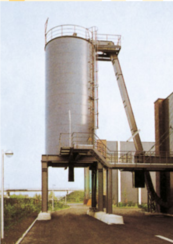
Truck loading silo for sludge cake
