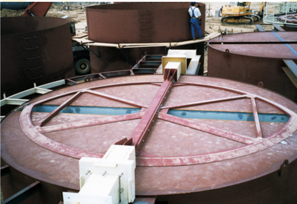
Installation of tandem Sliding Frame for wood material in 6000 mm diameter silo during silo construction.
